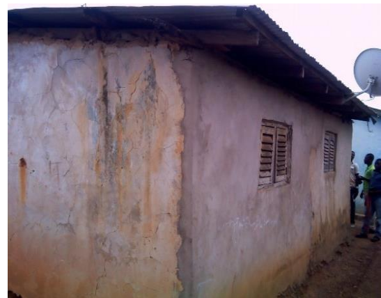
Fig. 6 47-Year Sun-Dried Brick Structure rendered with Cement Mortar (Structure has multiple cracks and no foundation)
