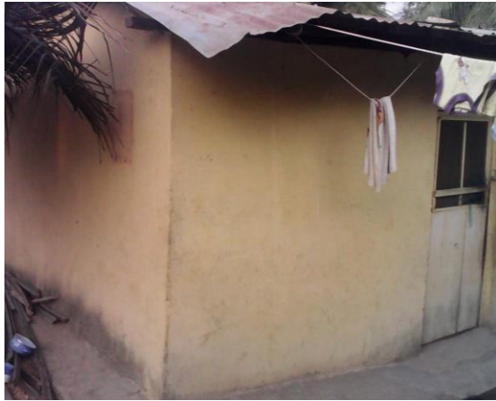
Fig. 7 19-Year Old Wattle and Daub rendered with Cement Mortar (Structure has no cracks)
