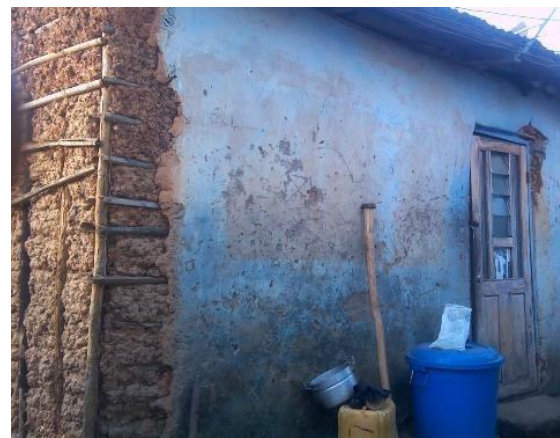
Fig. 5 21-Year Wattle and Daub Structure partly rendered with Cement Mortar (Structure shows multiple desiccation cracks)
