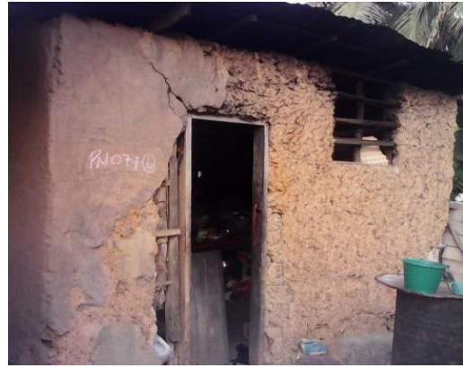
Fig. 4 32-Year Wattle and Daub Building partly rendered with Clay (Structure has multiple cracks and no foundation)
