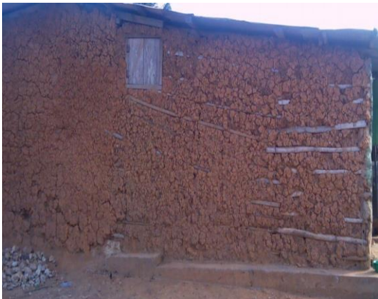
Fig. 3 20-Year Old Wattle and Daub (with multiple desiccation cracks)
